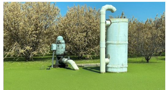
GAR Bennett creates, installs and helps growers maintain the most efficient system for their crops.
