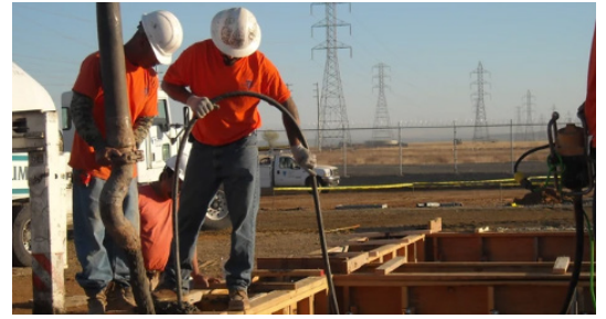
Pictured is the Arrow Construction SMUD Project, a Sub-Station in Rancho Cordova.
