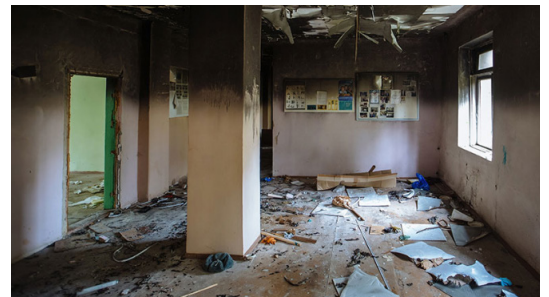
Restoration Management Company trains workers to restore properties back to occupiable condition following fire or smoke damage.
